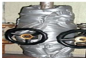
Valve heat insulation
